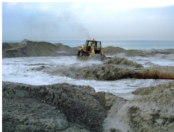
Figure 11. Sand and mud materials are pumped from a marine burrow area into the reclamation site. ‘Dyar Al Muharraq’ development in Bahrain- 2013 (Naser, 2014).
